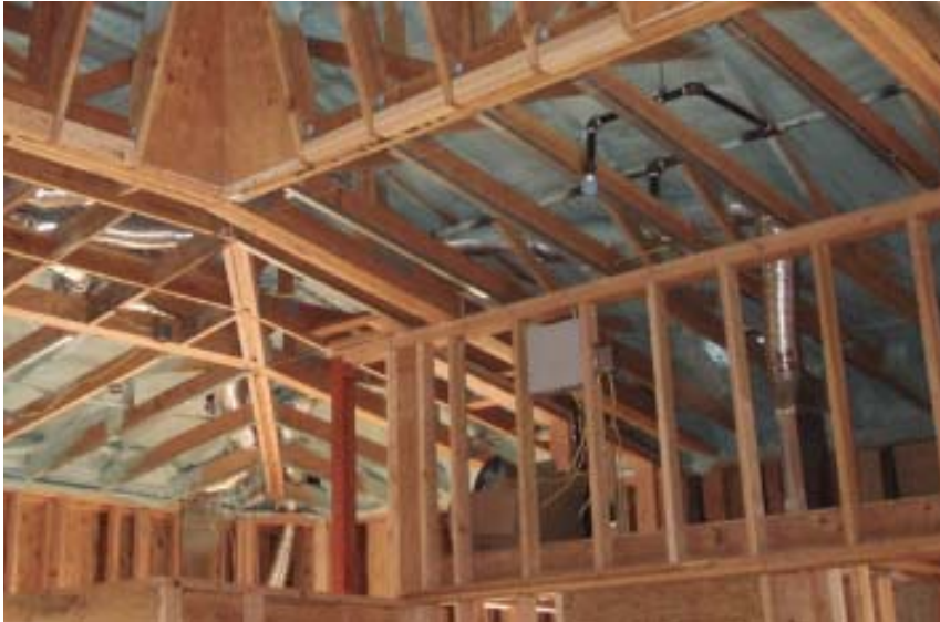
Figure 3. The ducts visible in this unvented attic will be concealed after drywall is installed. But because they are in conditioned space, they won't be subject to the extremes of temperature typical of attics.
